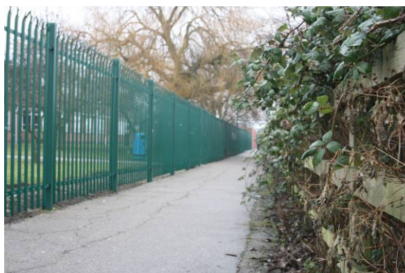
Overhanging vegetation around the boundary of the school
